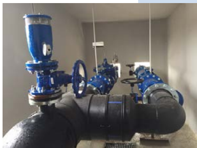
Spain Pump station
